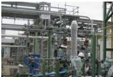
Siam Mitsui Wasterwater Plant
